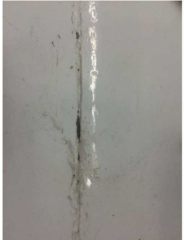
Figure 1: Exposed black primer on Gen 2 ESD floor from impact damage.
