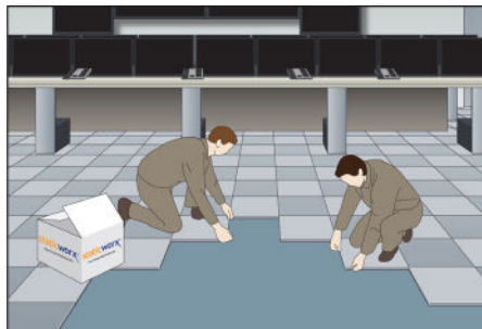
A low-charge-generating ESD floor is installed in the command center.
